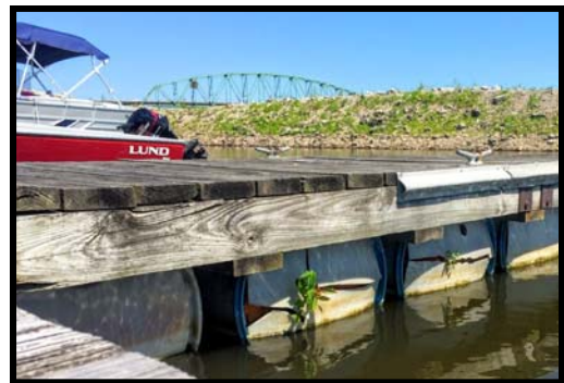
Floats Deteriorating at the Long Dock
