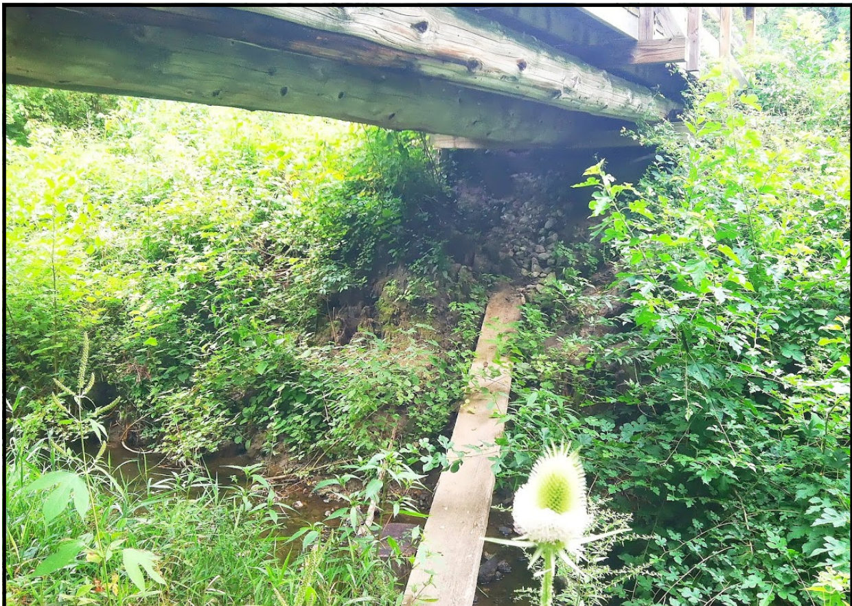
Erosion at Fuller Park
