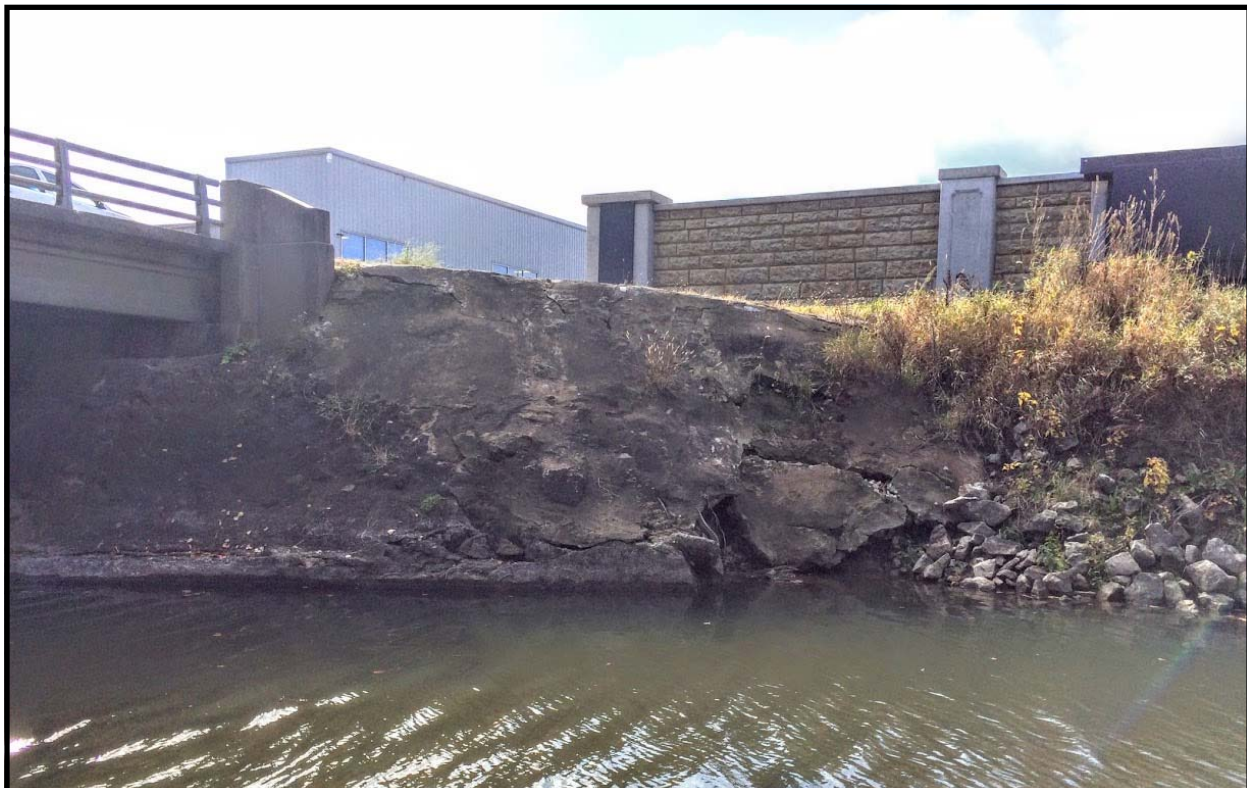
Scouring at the 2nd Street Bridge
