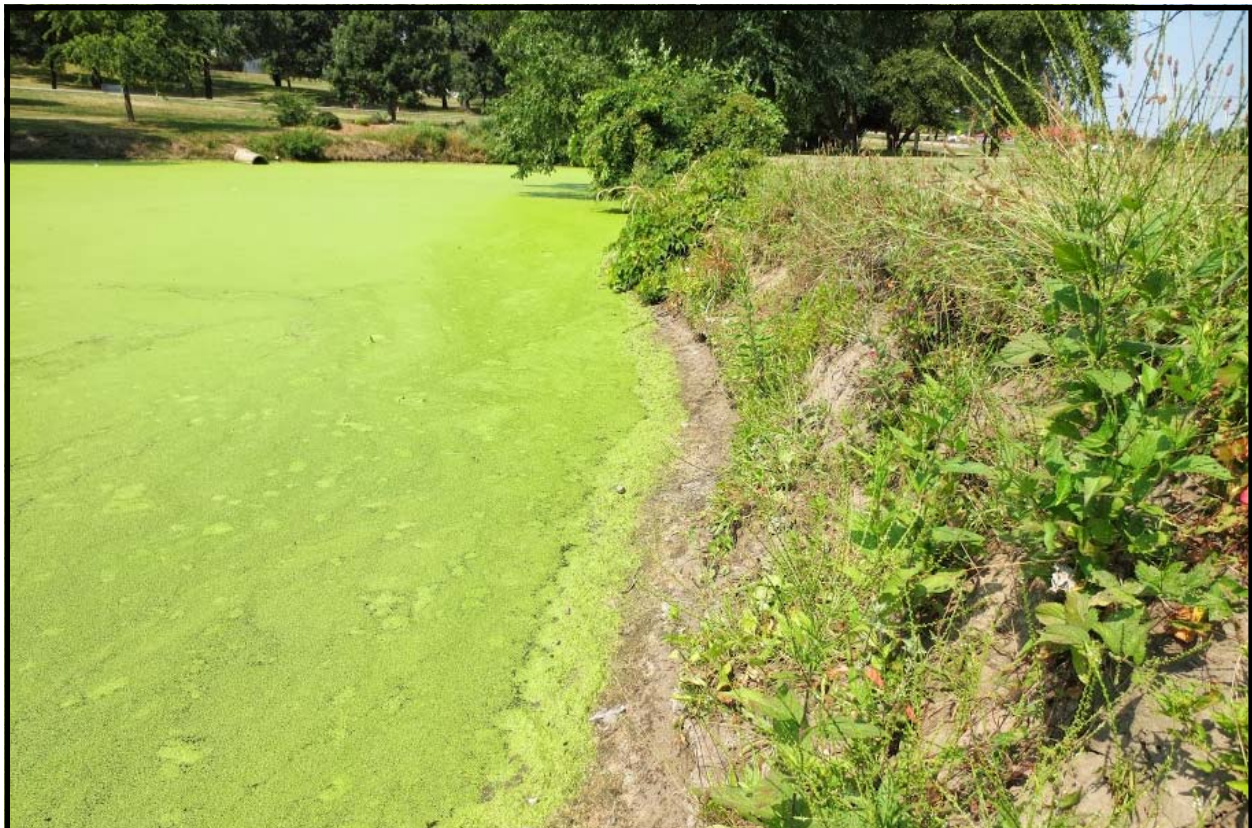
Erosion at the Weed Park Lagoon
