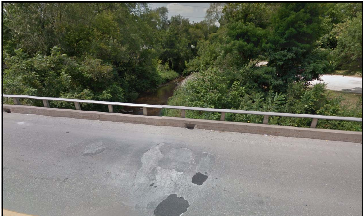
Scoring at the 2nd Street Bridge
