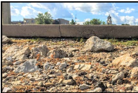
Erosion Beginning to Undermine Harbor Sidewalk
