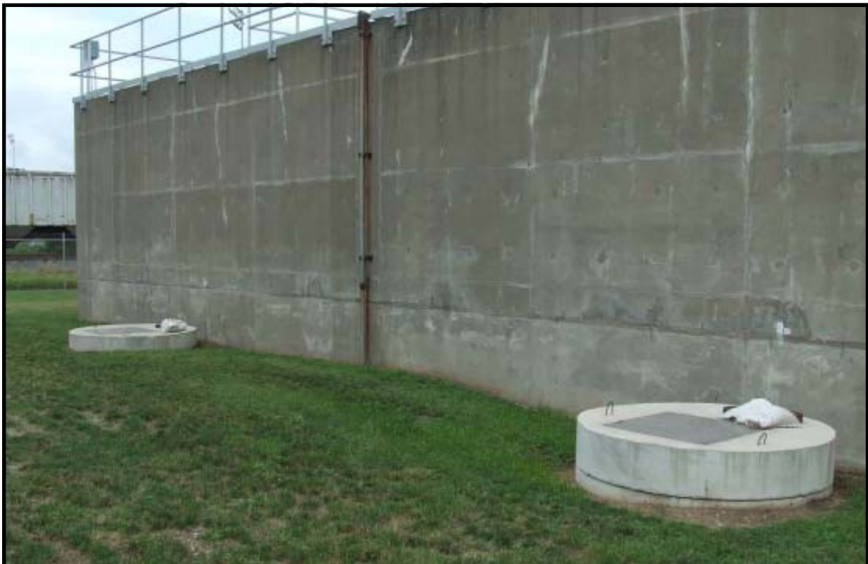
Figure X: Existing Quad Valves
